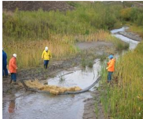
Sorbent and straw filter fence
